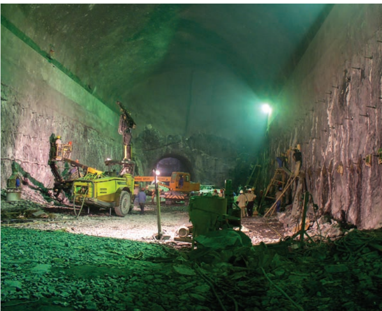
Above: Pumped storage projects call for many and varied underground excavations from tunnels, shafts and adits to caverns
