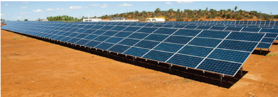
The solar power installation built by TransAlta Renewables at BHP's Northern Goldfields mine in Australia. CREDIT: STANTEC
